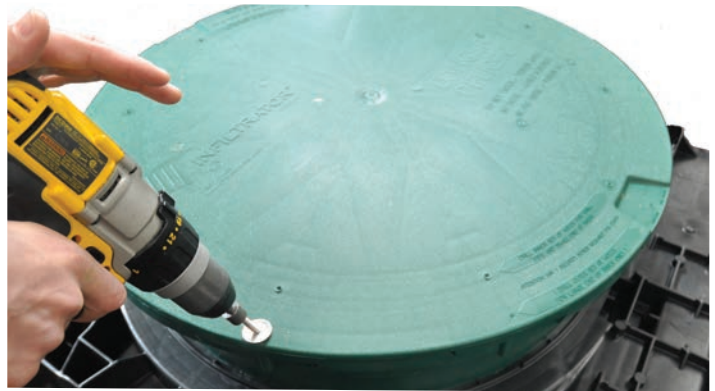
Prior to backfilling, fasten the lid to the riser with screws provided.
